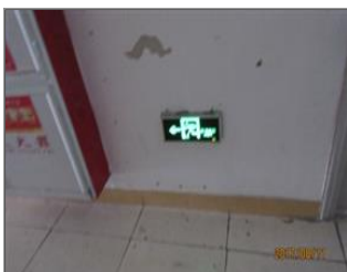
External photo(s) of the production unit(s) Evacuation sign in the dormitory.JPG
