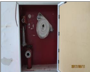
External photo(s) of the production unit(s) Fire hydrant in the dormitory.JPG
