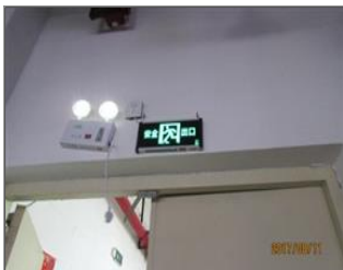
External photo(s) of the production unit(s) Emergency light testing.JPG
