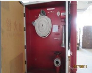
External photo(s) of the production unit(s) Fire hydrant in the workshop.JPG
