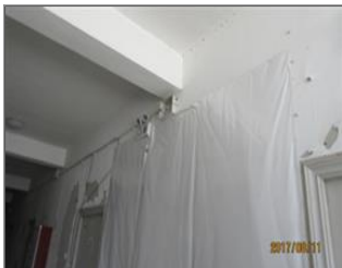
External photo(s) of the production unit(s) Emergency light in the dormitory.JPG
