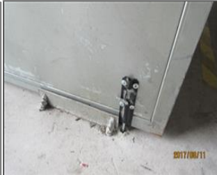
External photo(s) of the production unit(s) NC 7.15 Remark Locking device installed at the sliding door to keep opening durign working time 1.JPG
